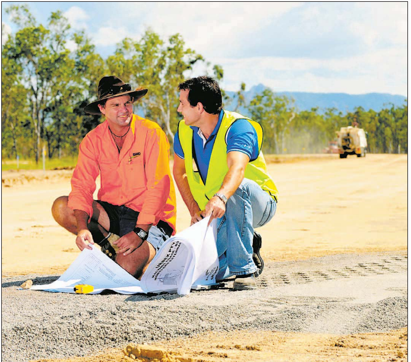
JOURNEY: Kalynda Chase, Aidan Geaney Project manager and John Barron Site foreman for BMD Construction at the site where a new road being built to connect Kalynda to the Ring Road.
