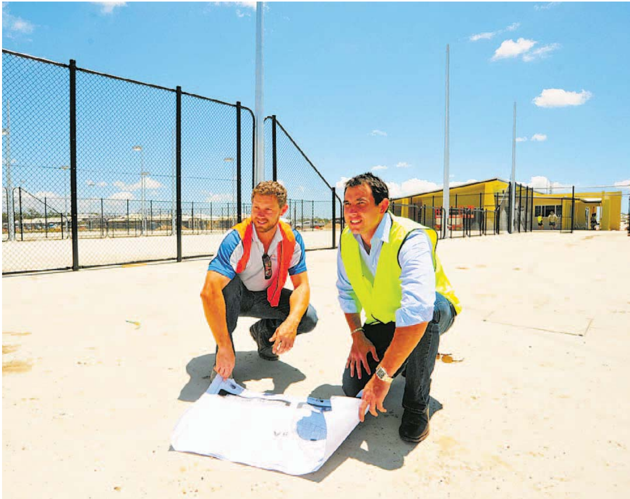
TAKING SHAPE . . . Oliver Loughlin, Court Craft project manager and Aiden Geaney project manager at Kalynda Chase tennis centre and club house
